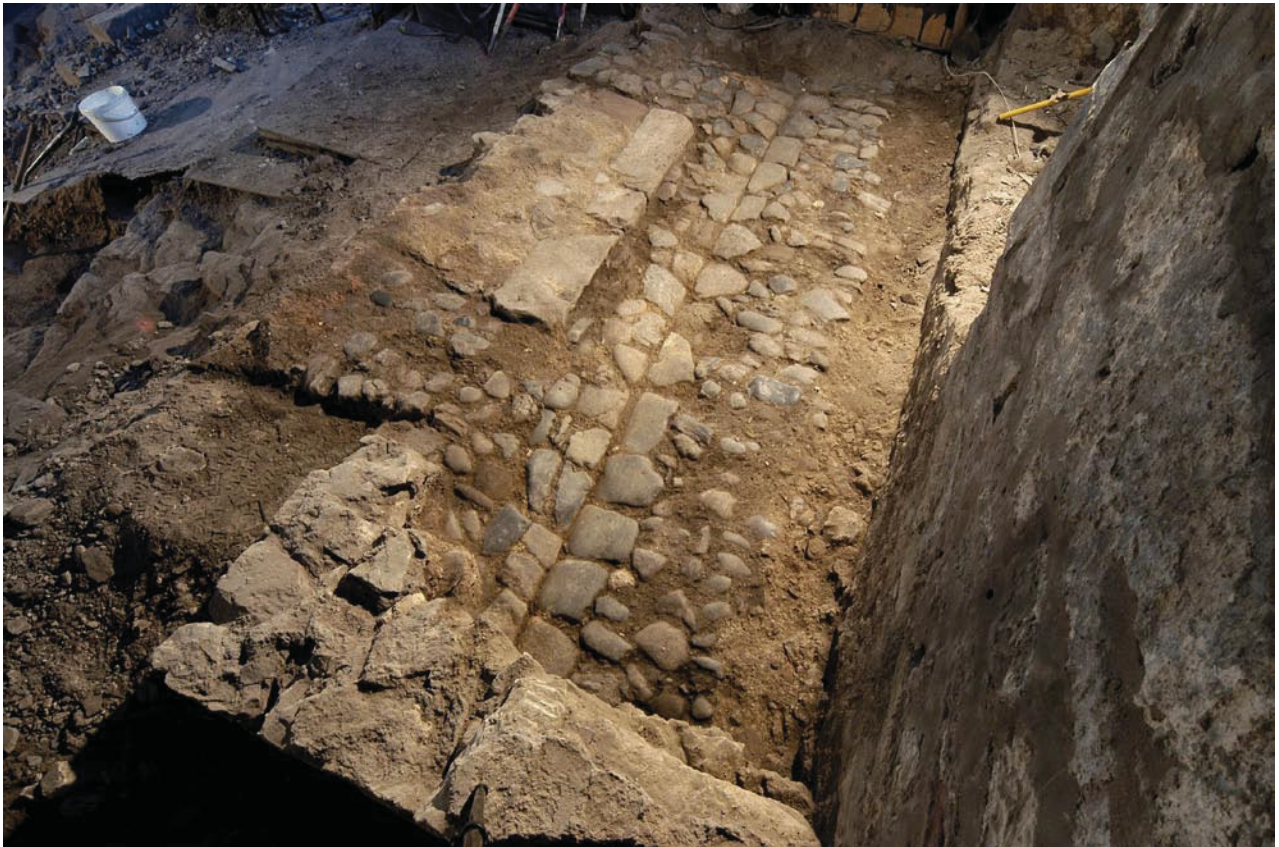
Illus 5 Work in progress in the Tron Kirk. Marlin's Wynd is the cobbled street running from the foreground north towards the High Street.
