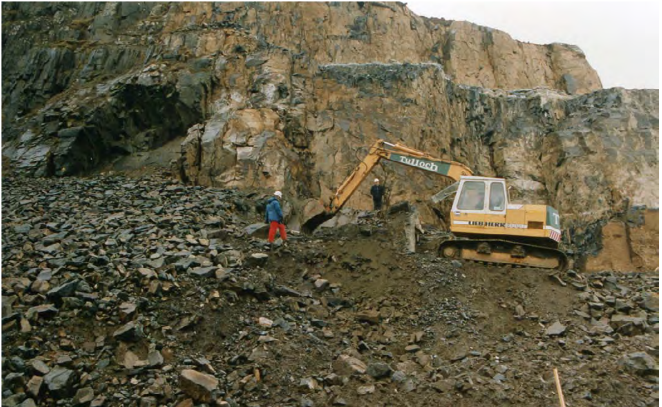
Illus 10 Rock clearance in progress in 1994 viewed from the east following the rockface blasting (photo: Roger Miket)
