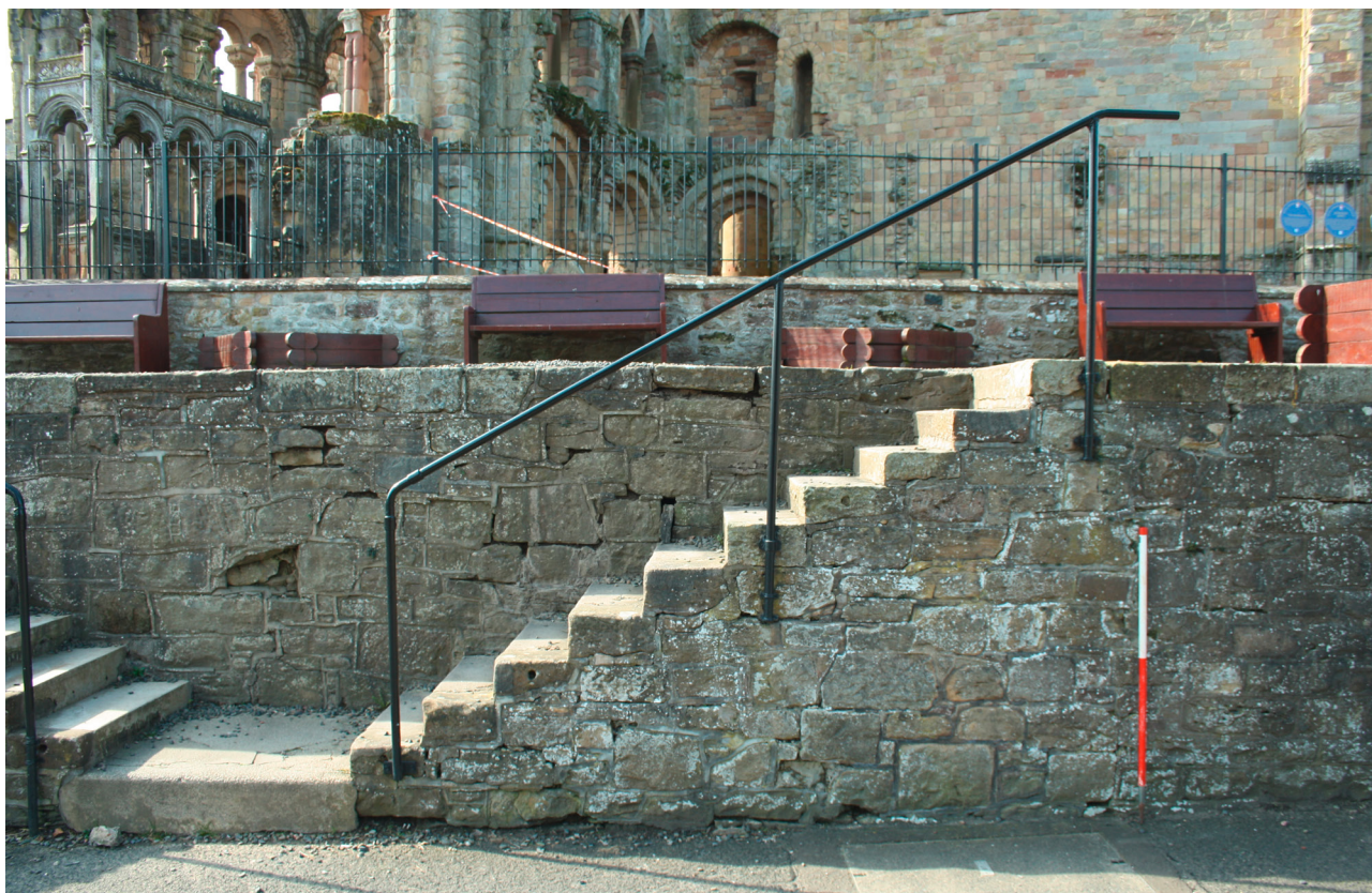
Illus 5 Photograph showing failure and damage to ‘rampart’ wall at former double access steps (Image by Heritage and Archaeological Research Practice)
