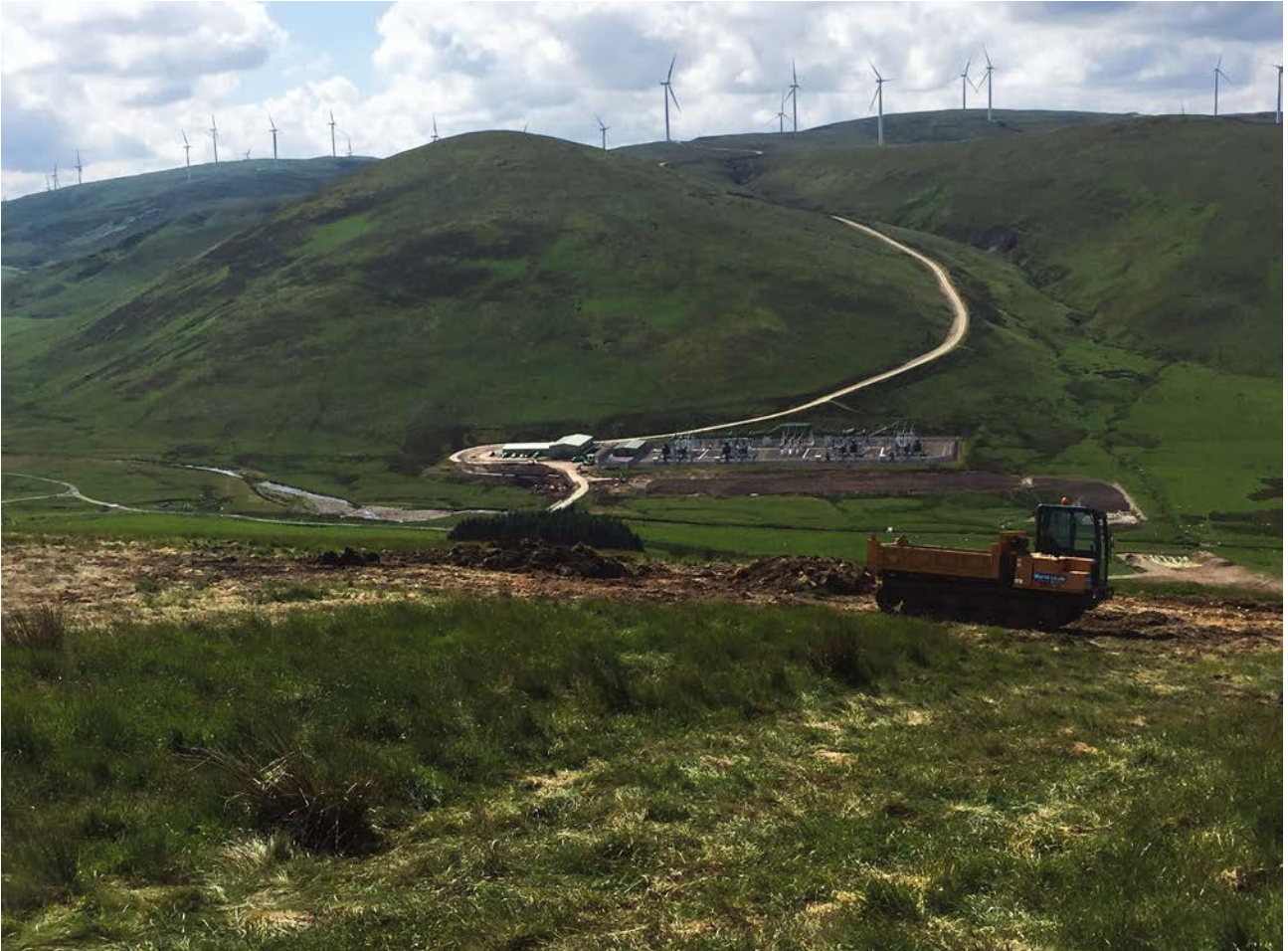
Illus 7.5 Midlock Valley during construction of the cable access route. (© Headland Archaeology (UK) Ltd)
