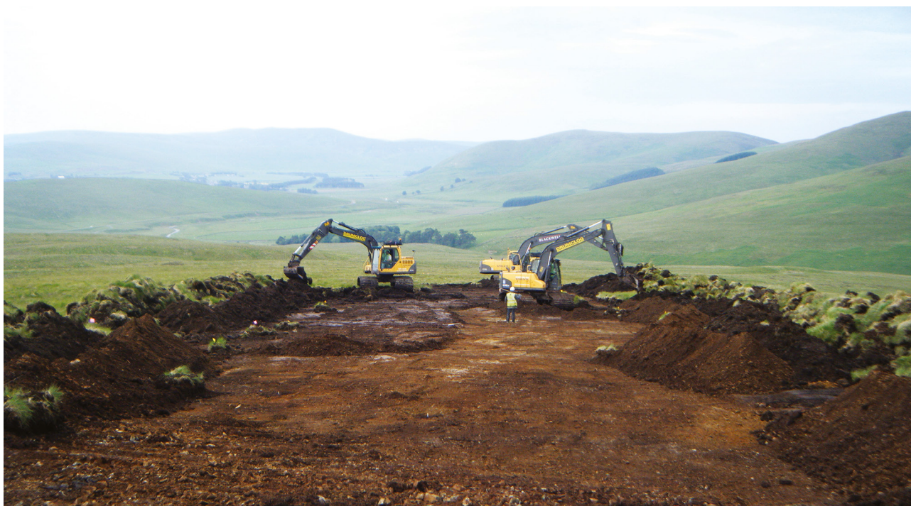
Illus 7.1 View of topsoil stripping for access road on northern side of Camps Valley. This provides a typical view of the landscape of the wind farm. (© Headland Archaeology (UK) Ltd)(© Headland Archaeology (UK) Ltd)
