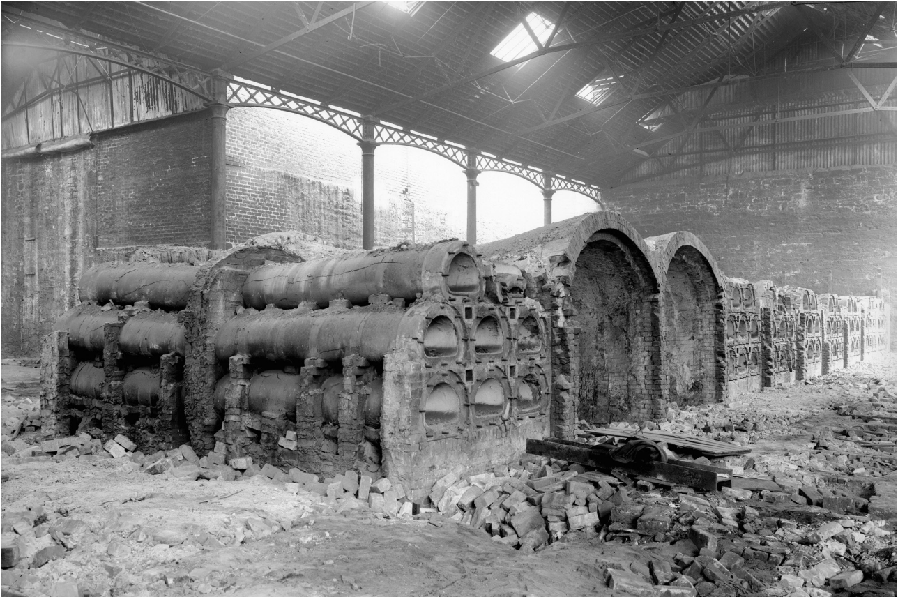
Illus 12 Horizontal retort benches and double furnace in process of demolition (© HES)
