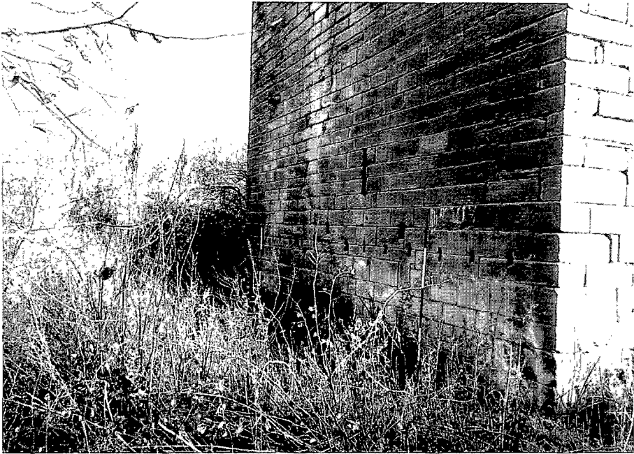
ILLUS 7 The north face of the tower showing timber sockets associated with at least one building formerly set against it
