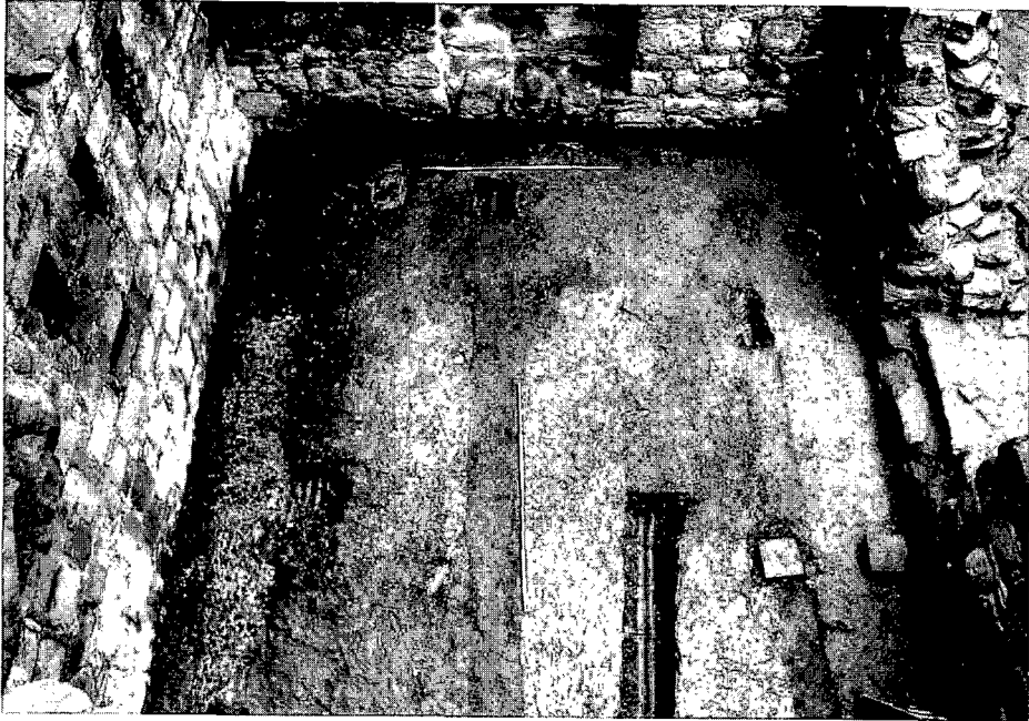
ILLUS 3 · The interior of the tower house, showing modern drains cutting the basement floor; viewed from the north
