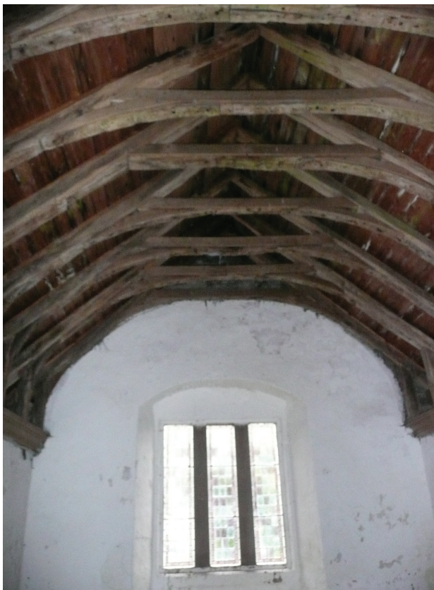
ILLUS 3 The Guthrie Aisle, Angus. The roof was built with small oak beams from Scandinavia, felled in and around 1464. Oak boards from the eastern Baltic had been used for the painted ceiling which was once lined the roof (© Scottish Church Heritage Ltd)
