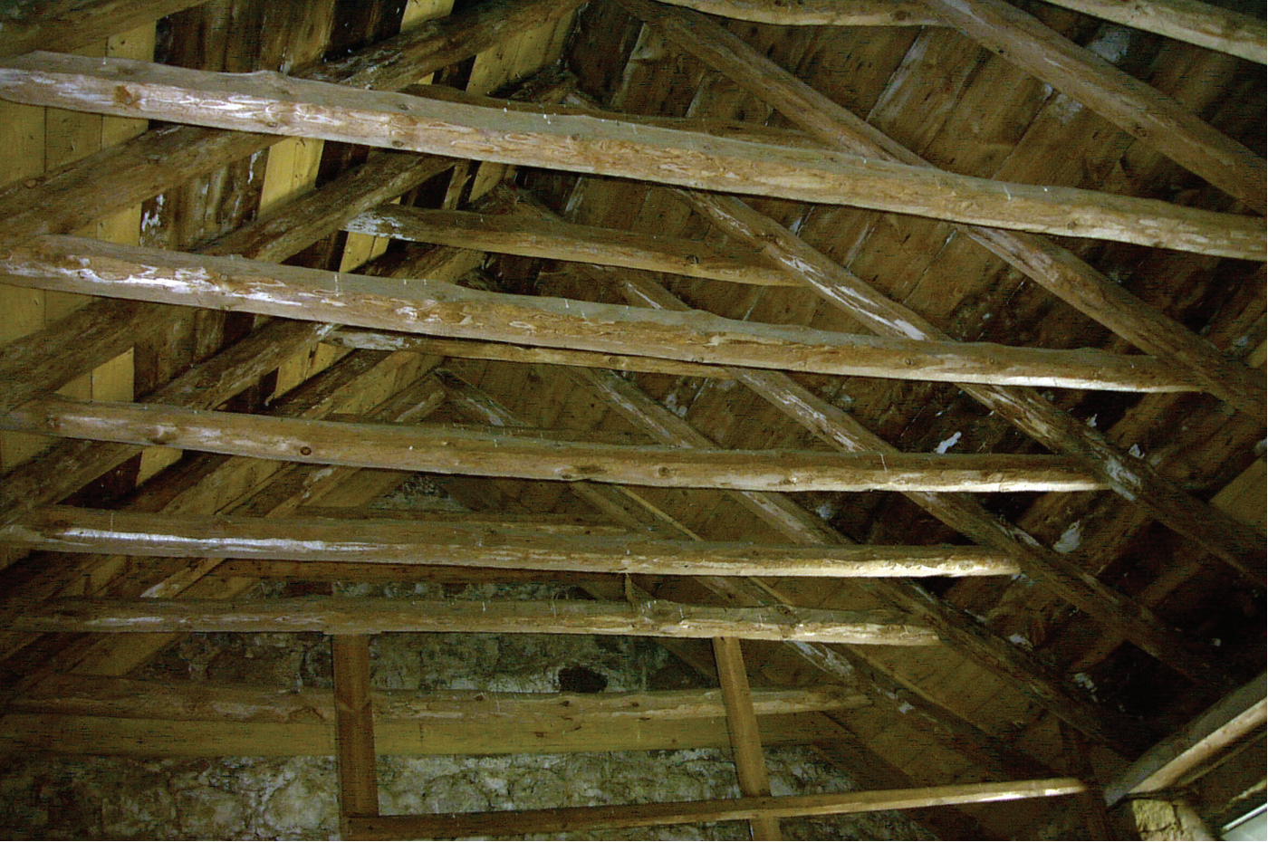
ILLUS 10 The Old Laundry, Drum Castle (c 1800). The roof has been built with small, fast-grown, hewn pine
