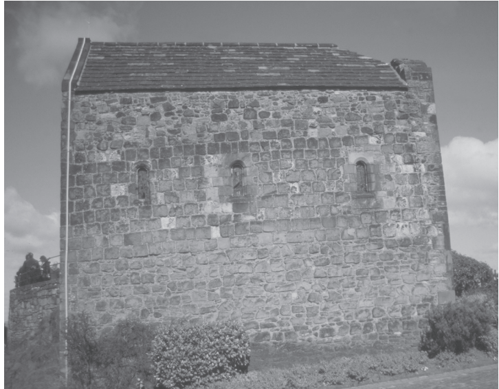
ILLUS 2 The south wall of St Margaret’s Chapel, Edinburgh Castle. Different styles of wall construction are clearly exhibited. Lower stonework represents underpinning but this gives way to ten regular courses of ‘cube-shaped’ stone. The lowest two courses of this stone show red colouration unlike the grey sandstone which comprises the higher eight courses. The more recently fabricated highest portion of the wall resembles the style of the underpinning in its construction
