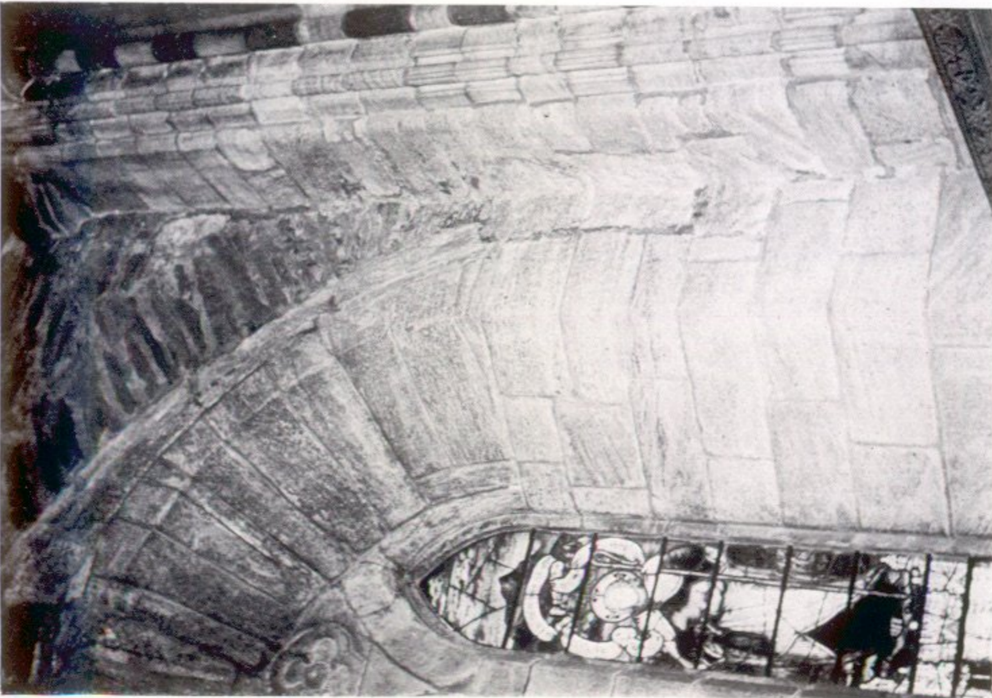
a Dunblane cathedral. Detail of masonry on S side of window at E end of S aisle
