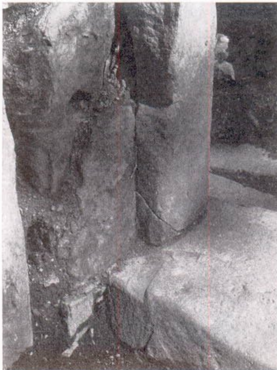
c South Tower, E jamb of entrance doorway showing step worn by Yett
