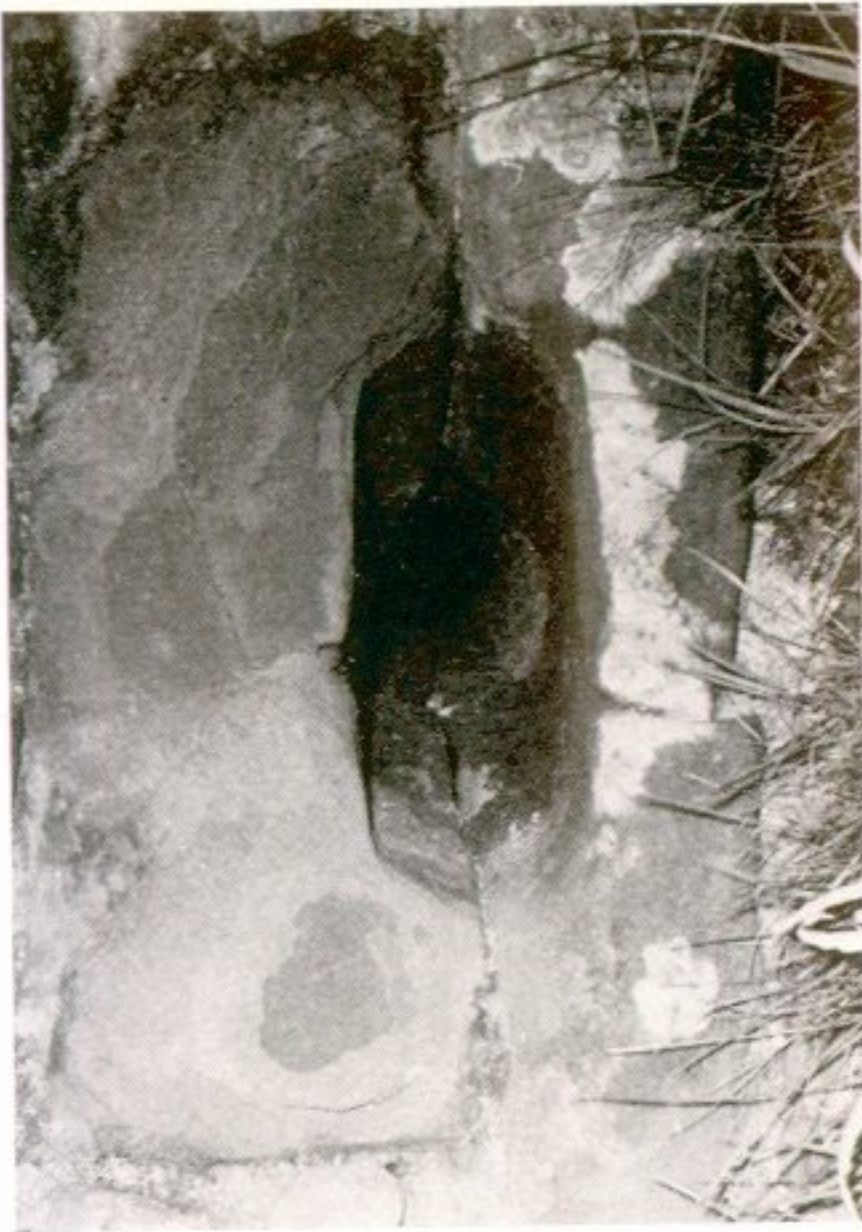
b Amisfield: splayed shot-hole dressings inserted into outer face of existing slit window (late sixteenth century)
