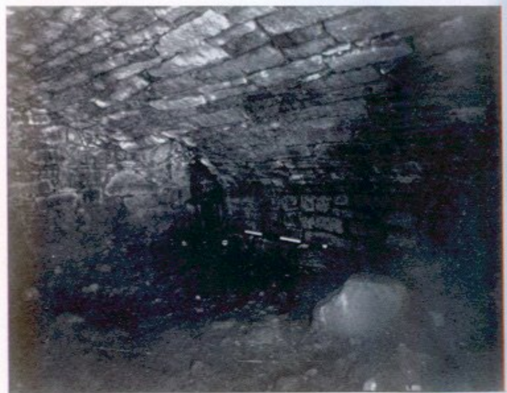
4. Finavon Castle: cellar in base of High Tower, showing 16th-century vault benched into face-work of 14th-century Great Tower.
