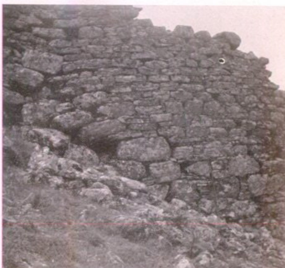
3. Dun Grugaig: masonry on southern arc, showing displacement of courses by subsidence.
