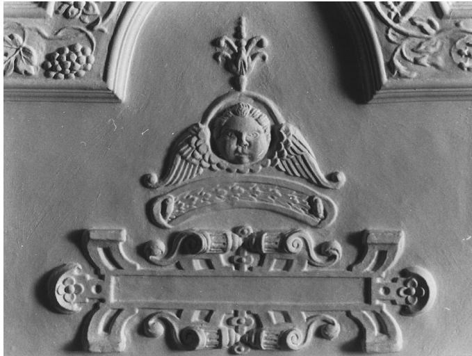
ILLUS 4 Cherub head with section of border from a roundel on the great chamber ceiling at Mapledurham. (Photograph by Richard Gapper, © Claire Gapper)
