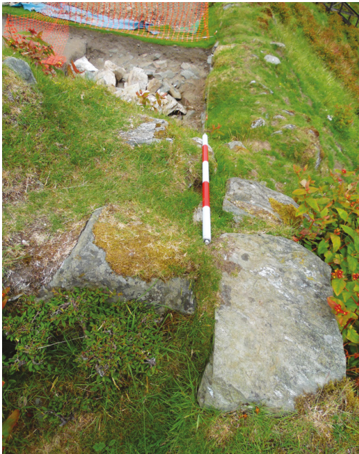
ILLUS 6 Straight Joint 1 from the south-west; highlighting continuity of the south-east curtain wall (right-hand side) and abutting cross-wall (left). (© Mark Thacker)
