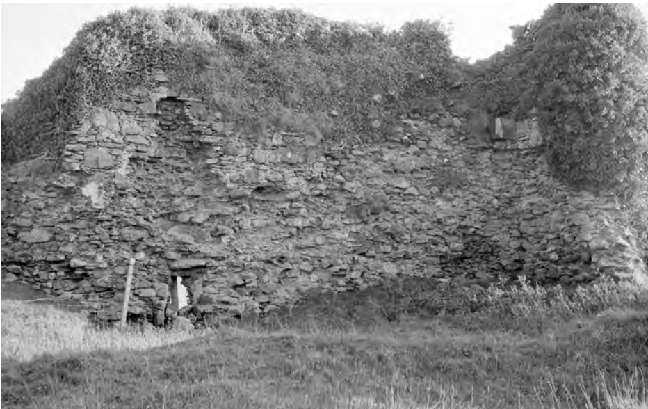
ILLUS 7 The south-east range from the north-west, 1964. Highlighting the almost complete loss of internal facing from upstanding south-east and south-west walls, and the extensive exposure of lime-bonded core rubble. (SC_1554986 © Crown Copyright: Historic Environment Scotland (Scottish National Buildings Record))
