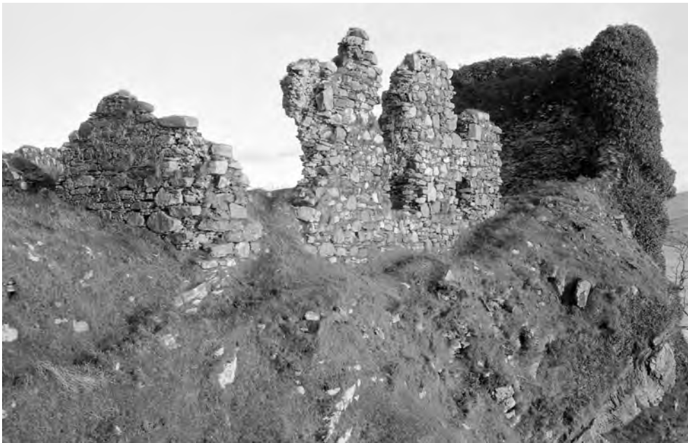
ILLUS 4 Castle Camus from the west; 1964. Highlighting the ivy-covered remains of the south-east range in the background and the south-west range in the foreground. The south-west range had suffered further significant collapses by the time of the current work. (SC_1554980 © Crown Copyright: Historic Environment Scotland (Scottish National Buildings Record))
