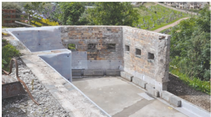
ILLUS 10 The surviving blockhouse at Kinghorn/Pettycur, partially demolished and being incorporated into a modern building, 2016 (Authors)
