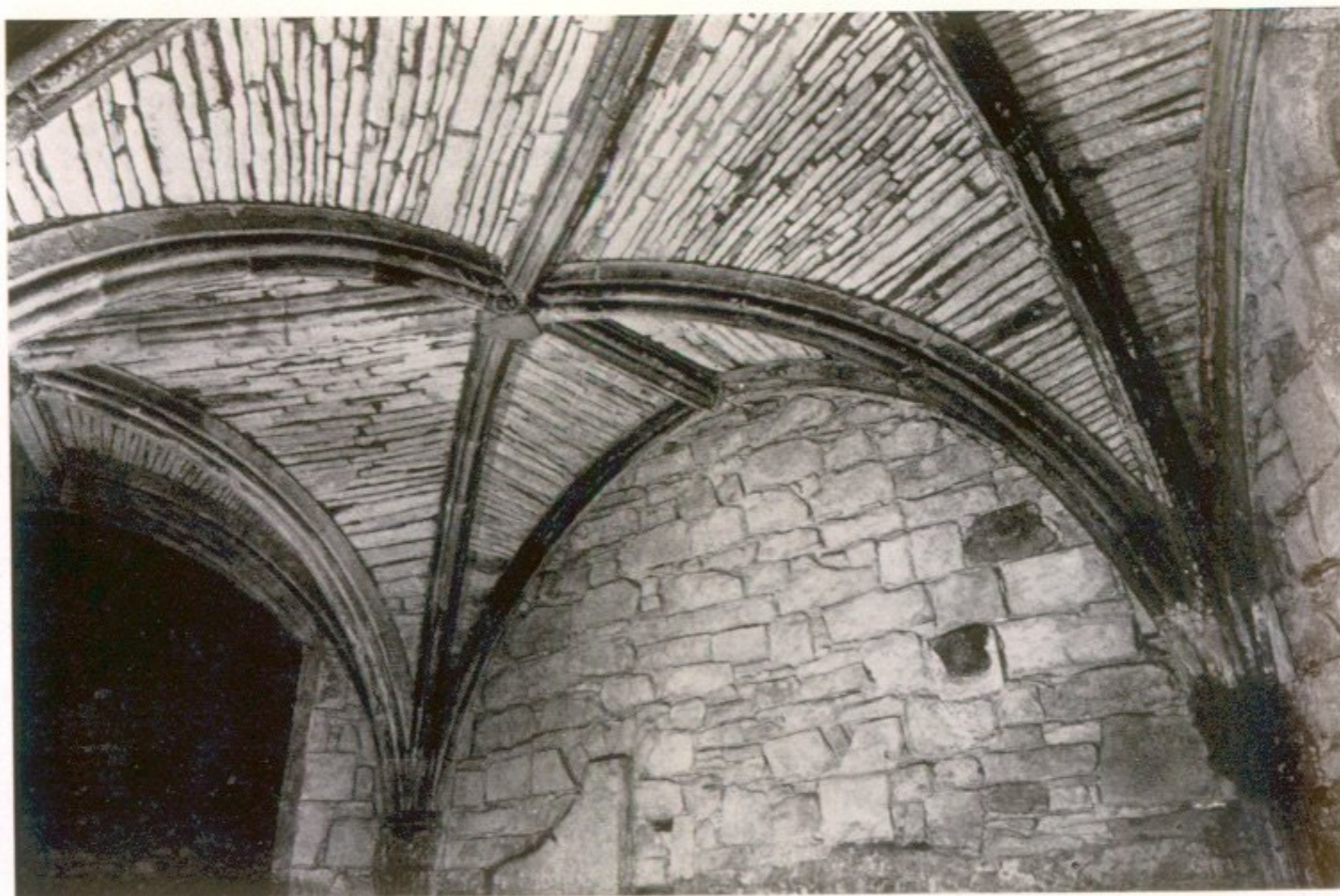
1. Lower chamber of hexagon: vault. Interior stripped of harling and consolidated by Ministry of Works
