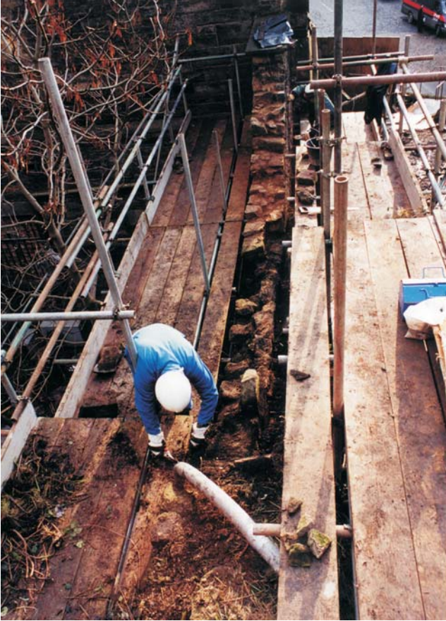
Illus 3 Working shot along the top of the Flodden Wall and the Phase 2 & 3 walls, facing south at the south-east corner of the Dance Base site
