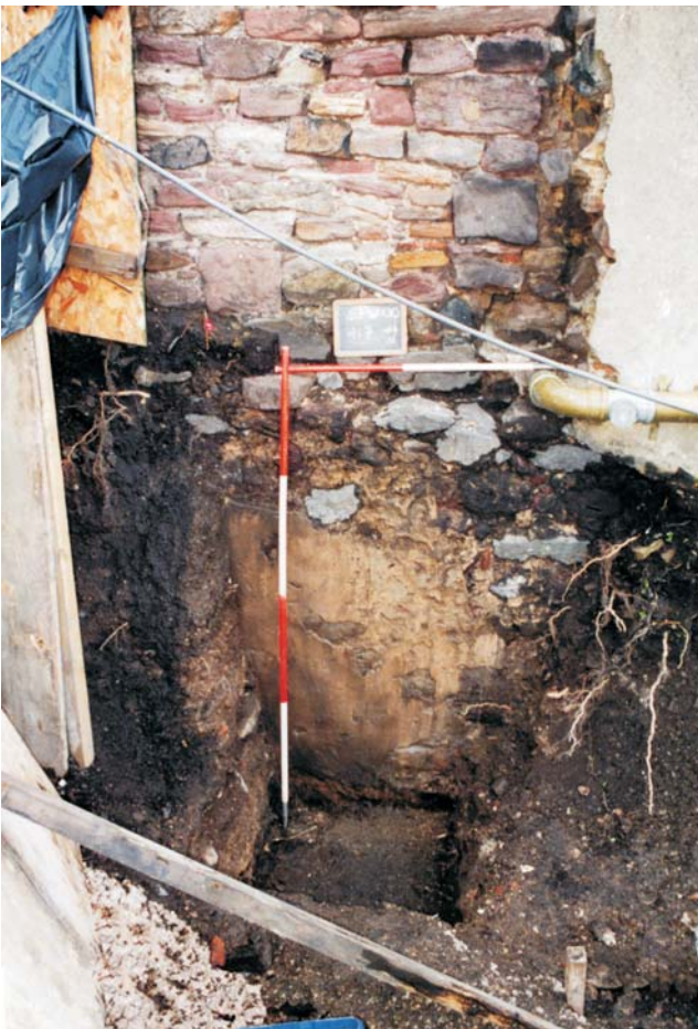
Illus 6 West-facing elevation of the Flodden Wall and the Phase 2 & 3 walls, showing Test-Pit C
