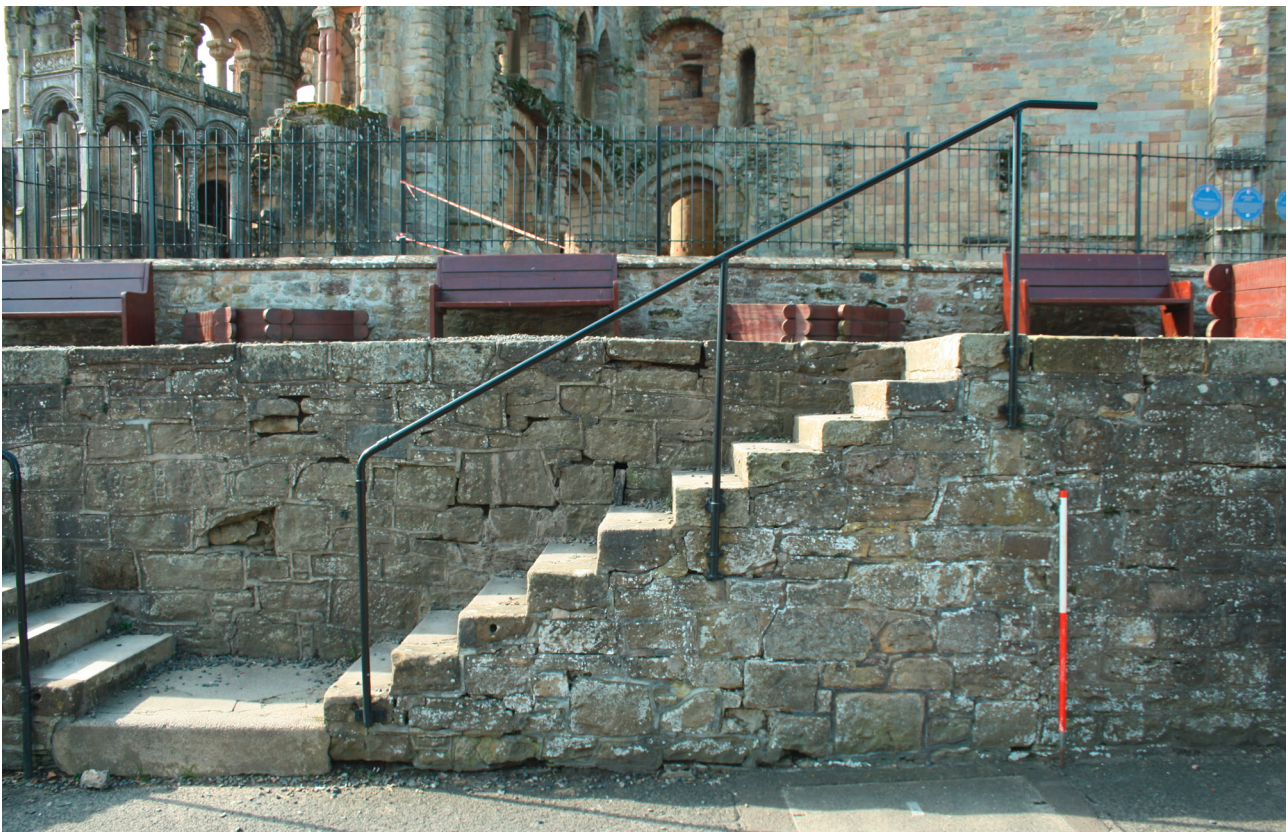
Illus 5 Photograph showing failure and damage to ‘rampart’ wall at former double access steps (Image by Heritage and Archaeological Research Practice)
