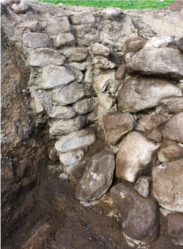
Illus 13 Detail of souterrain showing the cross-wall abutting the original side wall, facing west
