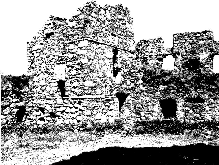
ILLUS 5 The great staircase from the west abutting the east wing. Note the Royal Arms of 1603 and missing lintel into the principal doorway. Note also the regularity of the windows in the east wing. (RCAHMS).
